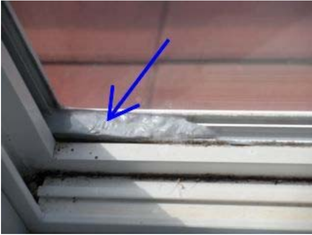
Photo 11 Melted thermal sealant
