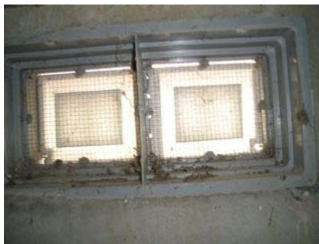
Photo 13 Blocked vent from crawl space
