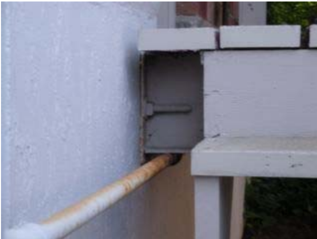
Photo 6 Gap between stairs and wall
