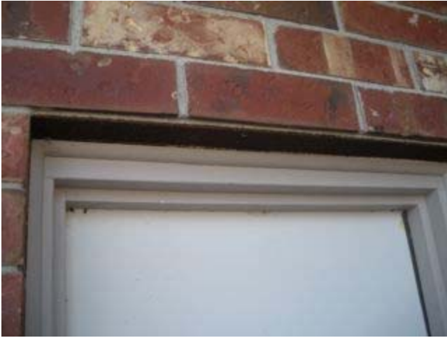
Photo 8 Rusted lintel plate
