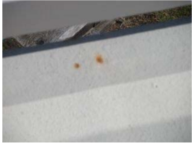
Photo 13 Rusted exposed nails on deck
