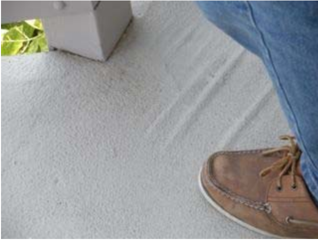
Photo 12 Buckled deck covering
